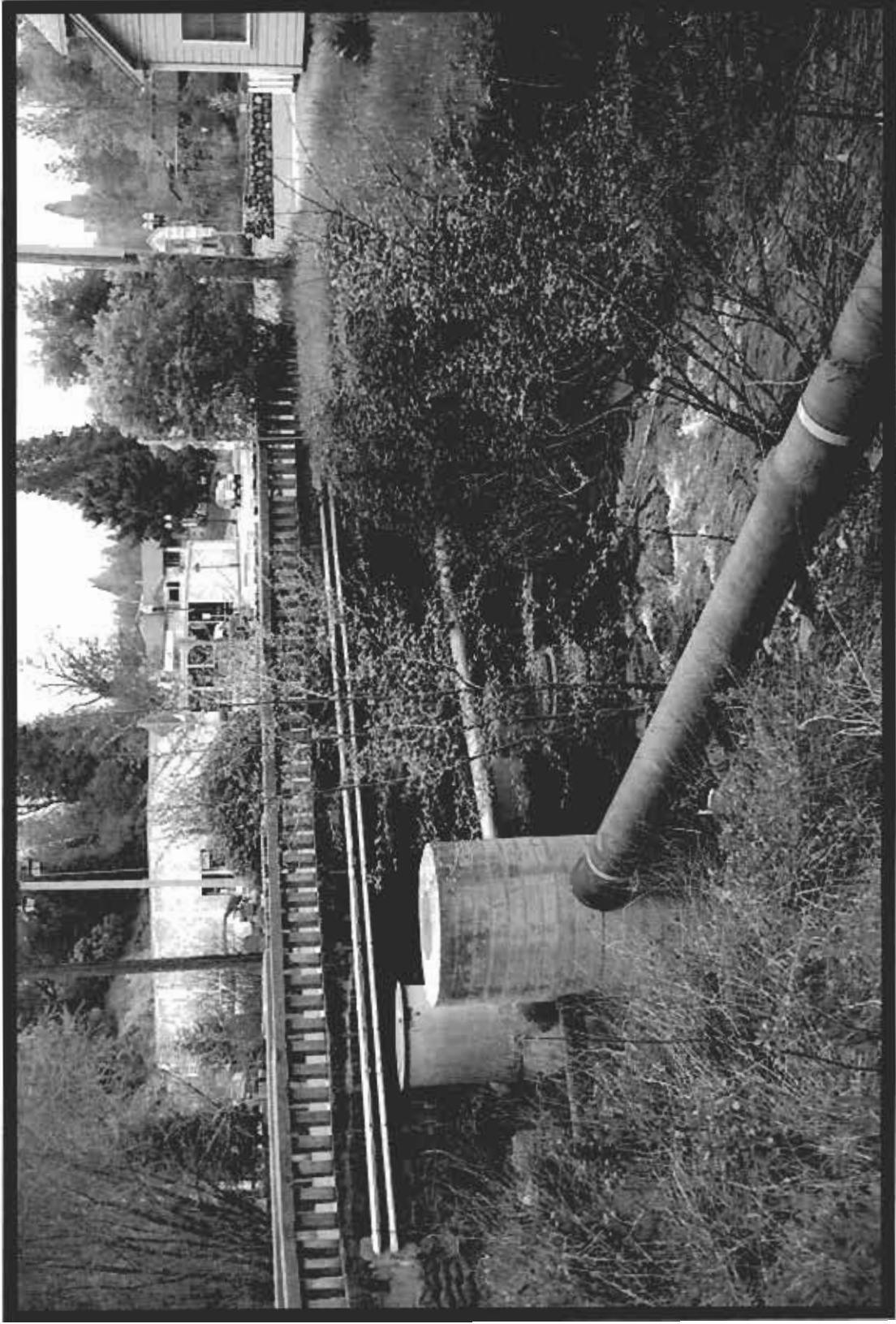
View facing southeast from near the northwest corner of the bridge. The Cedar Ravine culvert runs from the west side of Cedar Ravine, under main street, under the Ivy House parking lot to drain into Hangtown creek.
