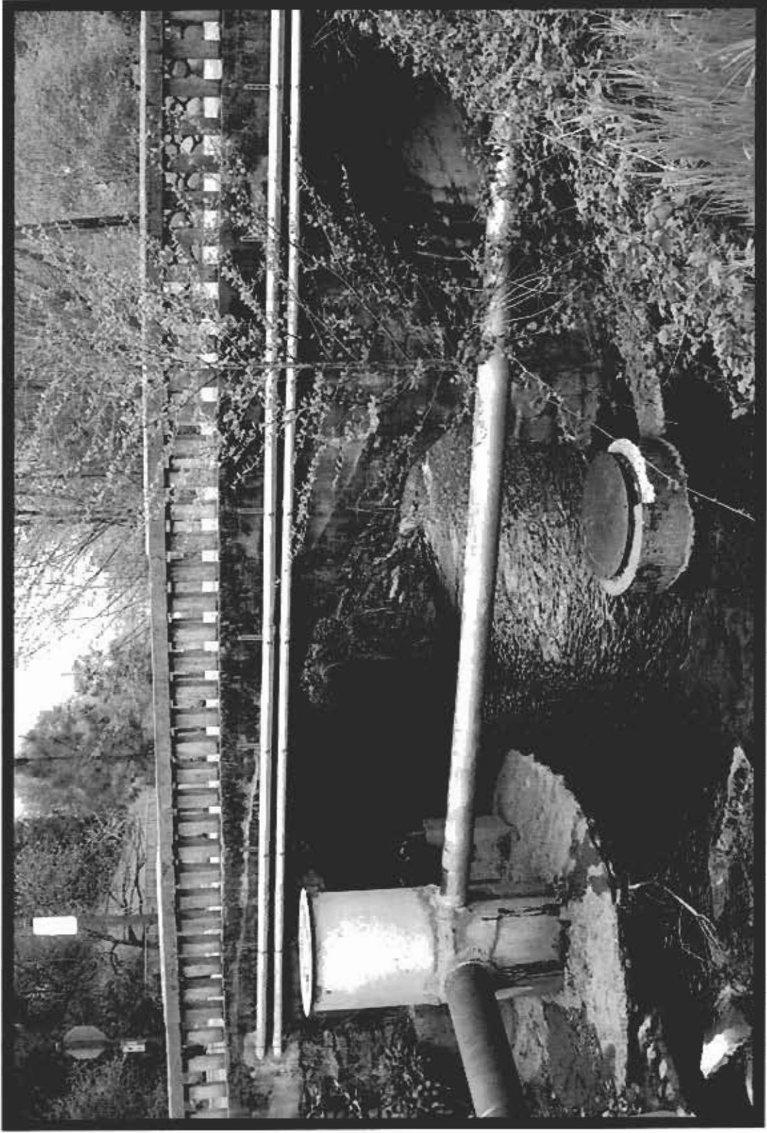
View facing east at the west side of the Clay street bridge. Notice the cedar ravine culvert draining into Hangtown creek through the southern abutment of the bridge. Also notice the new telephone line conduit hanging on the bridge that will be relocated with the proposed project.
